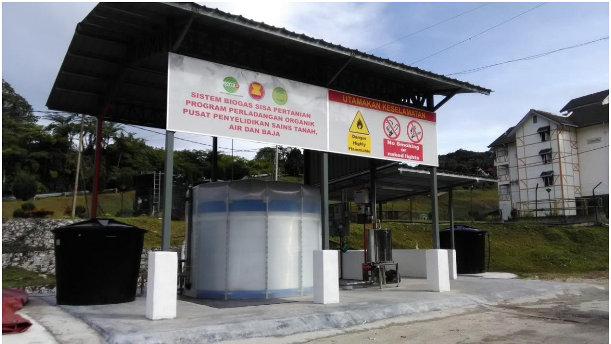
Figure 3: Biogas generator system have an engine capacity of 10kW
